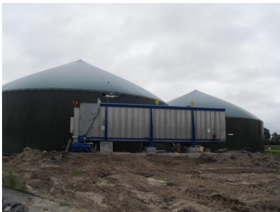
Solid material metering feeder 60 m 3 with screw press
